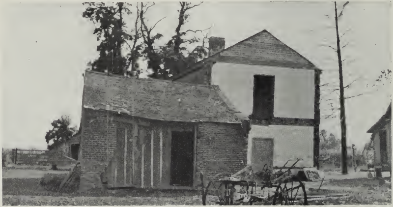
FIG. 42.—Brick house near Danville abandoned on account of danger by room-and-pillar mining of a 6-foot coal at a depth of about 200 feet.
